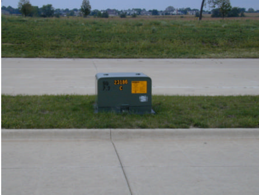
Attachment #3: Photograph of an electrical transformer cabinet.
