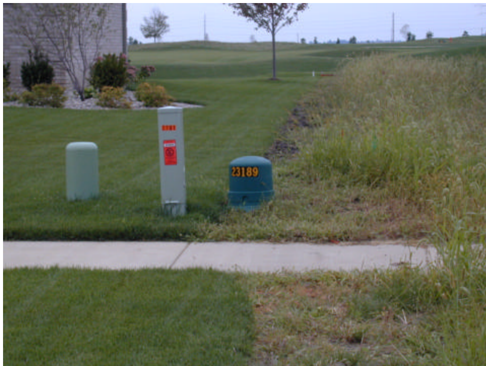
Attachment #6: Photograph of a cable, telephone and electrical pedestal. Cable pedestal shown on the far left.
