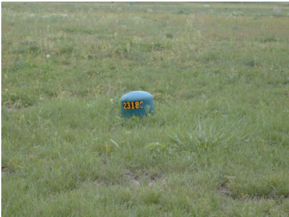
Attachment #4: Photograph of electrical pedestal.
