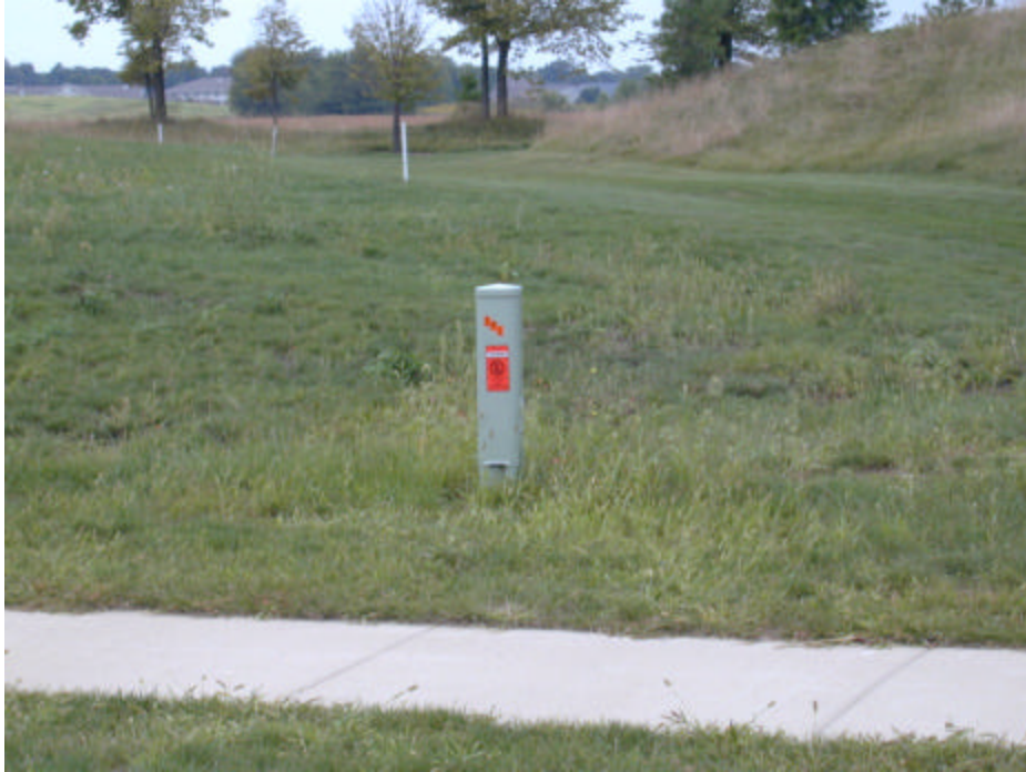
Attachment #5: Photograph of a telephone pedestal.
