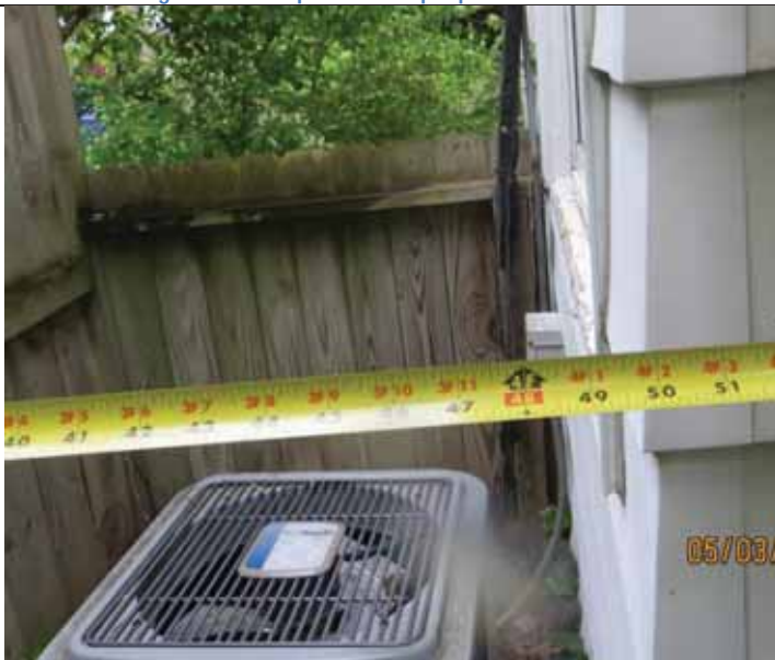
Figure 5. Measurement of side yard encroachment.
