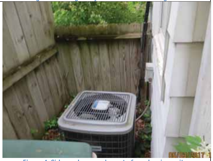
Figure 4. Side yard encroachment of condensing unit.
