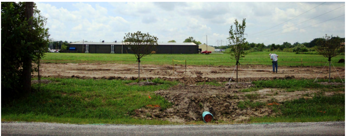
Subject parcel in foreground. Picture taken along Willow Rd., looking West. Photograph shows parking lot construction for building #2.
