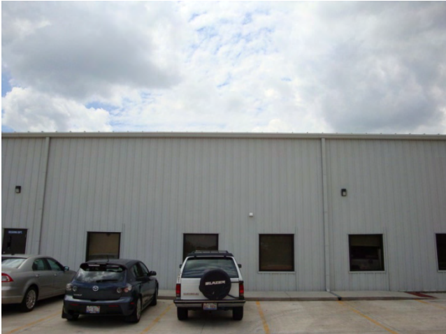
Existing CTS development, close up of East elevation showing use of aluminum windows and metal siding.
