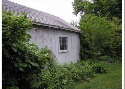
#10 East wall of garage on lot line from neighbors yard.
