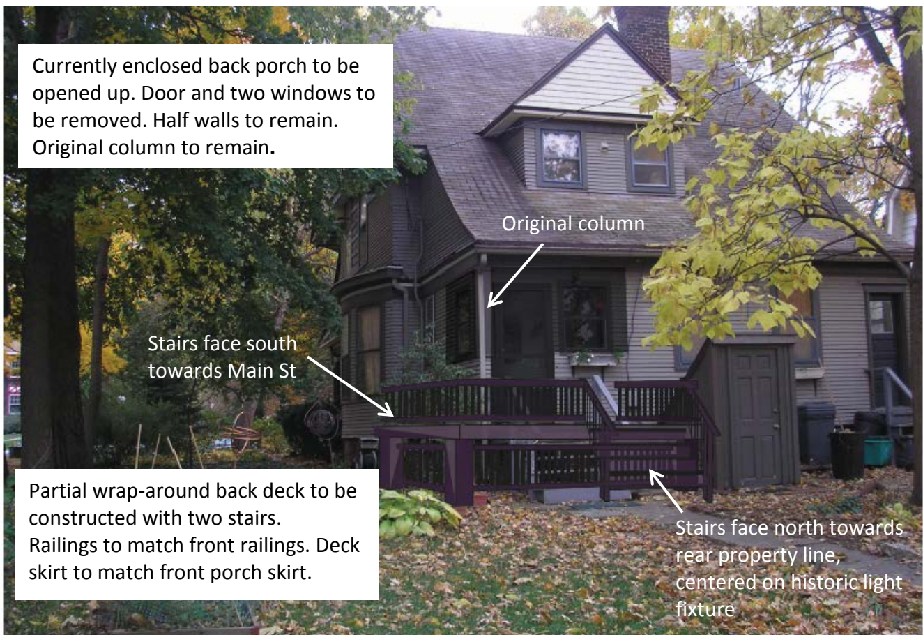
806 W Main St, rear elevation. City staff drew in the proposed deck and annotated this photograph to help the HPC visualize the proposed work.
