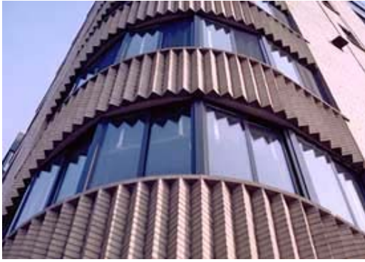
The historic steel sash has been removed and replaced with modern aluminum sash, resulting in a negative visual impact on the building's historic character. Photo: NPS files.
