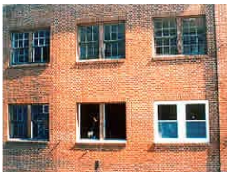
Inappropriate change to a historic building means the loss of its distinctive visual qualities, as well as a lessening of its long-term historical and cultural value. Photo: Martha L. Werenfels, AIA.
