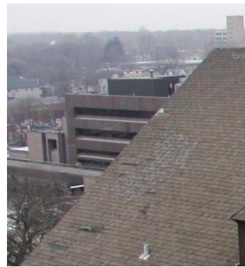
Close up of failing shingles
