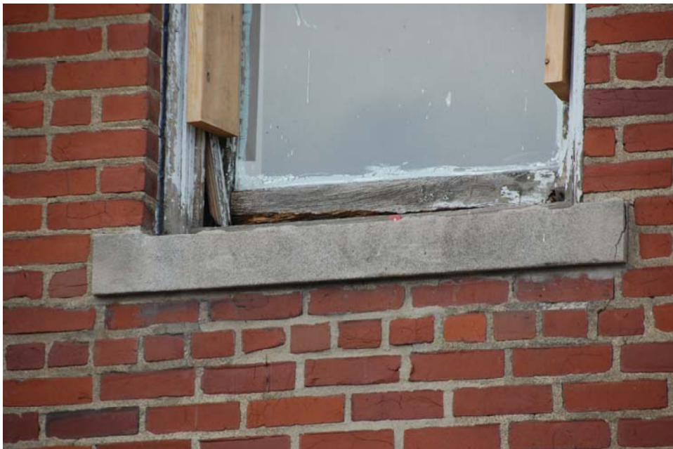
Notice rot along left side and along bottom rail
