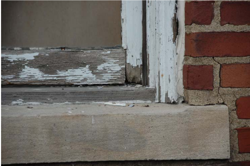
Most of the bottom portions of the frame and sash are rotted
