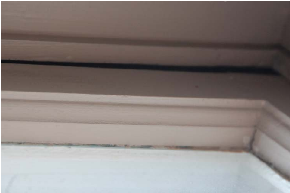
Top corner of 3rd-floor window with out-of-square frame
