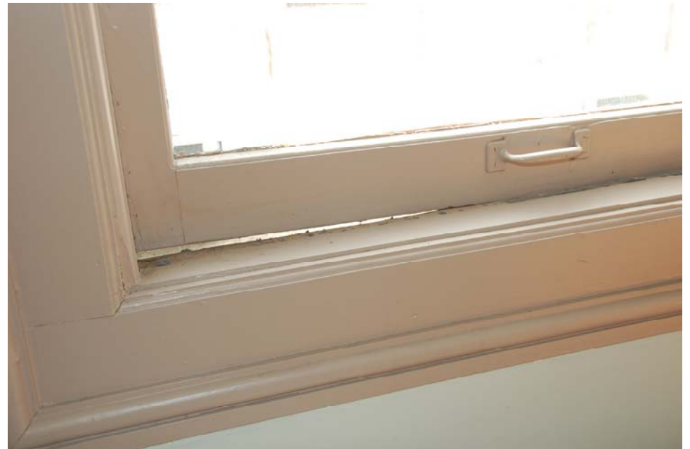
Lower corner of 3rd-floor west window with out-of-square frame
