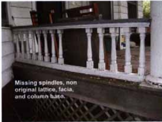
Porch Ceiling, missing end pieces, rotted overhang.
