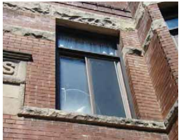
Left & Right: Deteriorated brick walls and windows at 218 W. Main.
