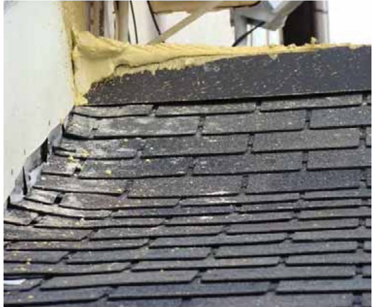
Above: Rafters and sheathing sagging beneath asphalt shingles at 201 S. Race.
