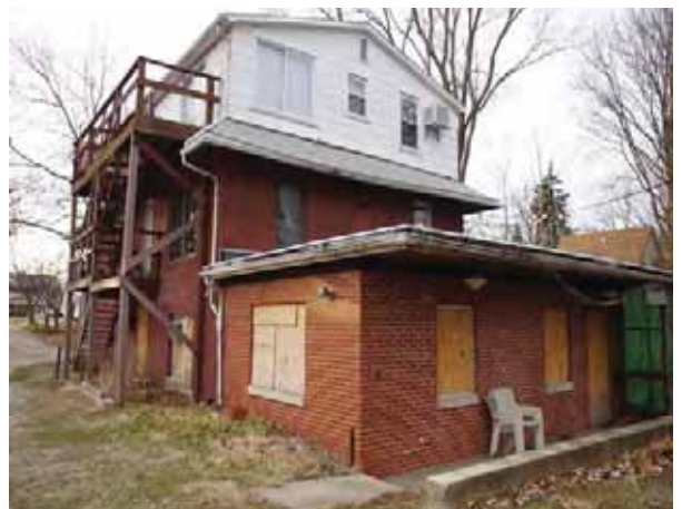
Right: 202 Wood is a deteriorated, boarded up multi-family apartment building with 1 occupied unit. This buildings has deteriorated siding, shingles and gutters. (03/07/2016)
