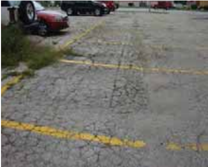
Above: The parking lot at 305 E. Main is deteriorated.
