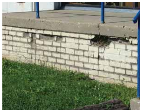
Right: A deteriorated brick front entry at 401 N. Broadway.
