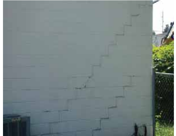
Right: Step cracking in the concrete block wall at 405 N. Broadway.
