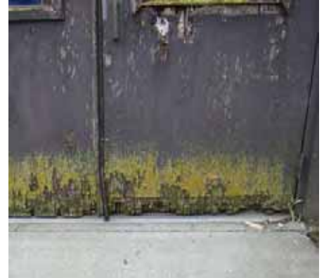
Above: The doorway to one of the halls at 201 S. Race is rotted and deteriorated.
