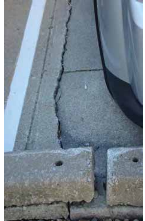
Above: A large shear crack, due to excess settling at 207 W Elm Street.
