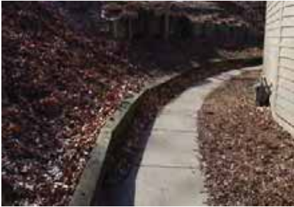
Left and Right: A leaning retaining wall located at Crystal Lake Park. (03/08/2016)
