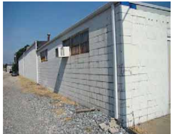
Right: A deteriorated exterior brick wall at 401 N. Broadway.
