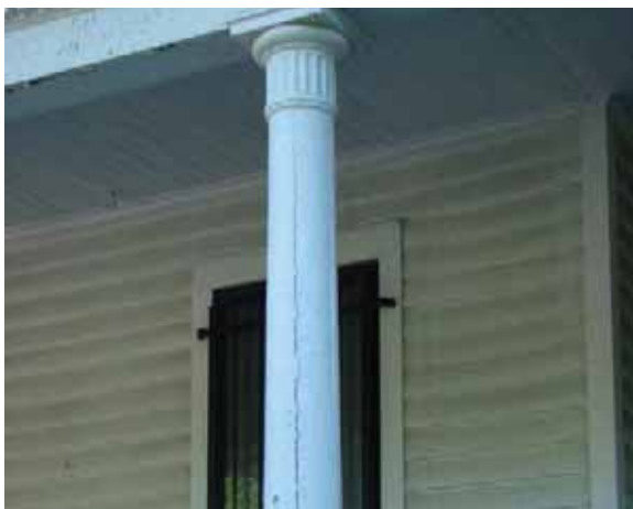
Left: The porch column at 206 S. Cedar is cracked.
