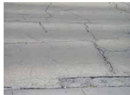
Above: Deteriorated pavement along Illinois Street.
