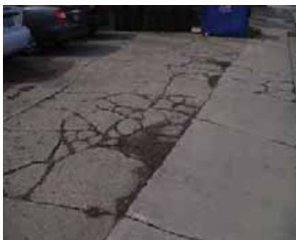
Left: The concrete parking lot at 101 W. Park is cracked and severely deteriorated. (03/08/2016)
