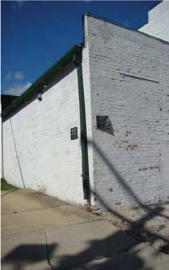
Left: The side wall at 208 W Griggs is also deteriorated.
