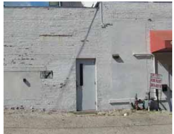
Right: A deteriorated exterior brick wall at 208 W. Griggs.
