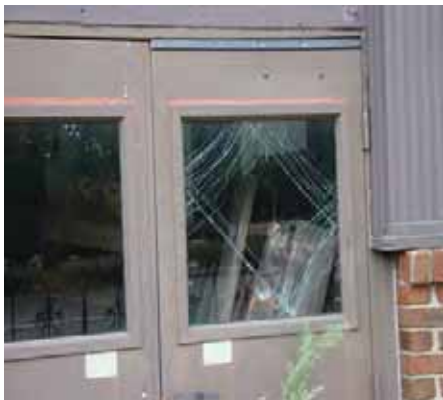
Left: A broken window on a side door at 201 S. Race.
