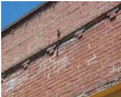
Below: The exterior brick wall at 130 W. Main is in need of tuck-pointing.
