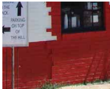
Above & Left: The exterior brick walls at 303 W. Main have severe step and sheer cracking.
