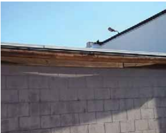
Left: A rusted and sagging gutter located at 201 W. Green.
