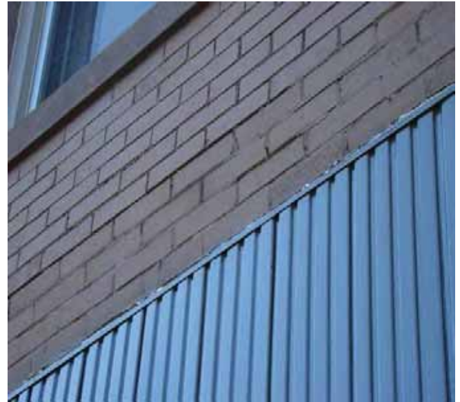
Above: A bulge in the exterior brick wall at 219 W. Main.
