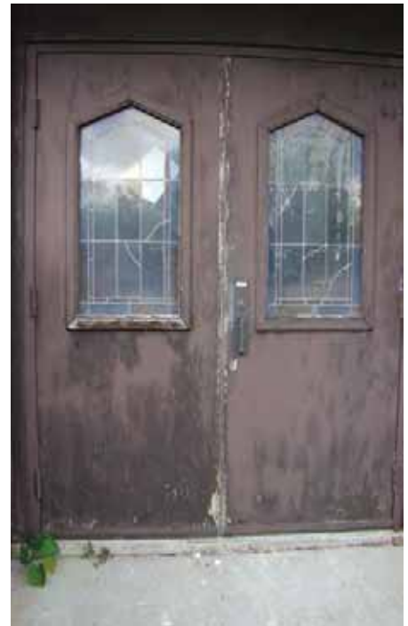
Right: A deteriorated door at 201 S. Race.
