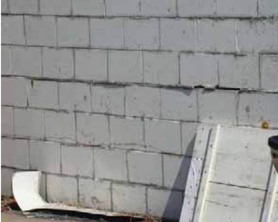
Left: Deteriorated mortar joints in the concrete block walls at 401 N. Broadway.
