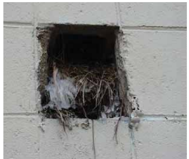
Right: A nest in an uncovered hole in the exterior wall at 207 E. Illinois.
