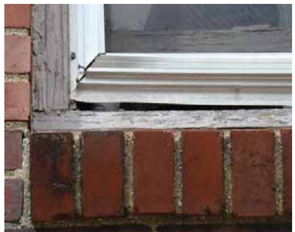
Right: The window frames at 402 S. Race are deteriorated.
