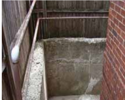
Above: Cracked and spalling concrete walls at 402 S. Race Street.
