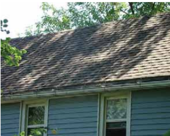
Left: The shingles on 404 N. Lake need to be replaced.
