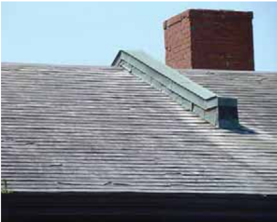
Left: The slate roof has cracked and missing shingles 403 W. University.
