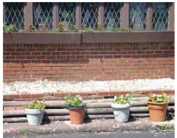
Right: 403 W. University is in need of tuck-pointing.
