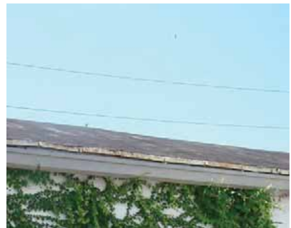
Right: The roof flashing on 302 N. Broadway is deteriorated.
