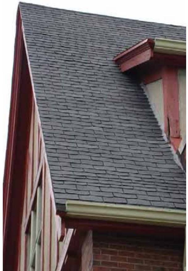
Right: The shingles on 402 S. Race are in need of replacement.
