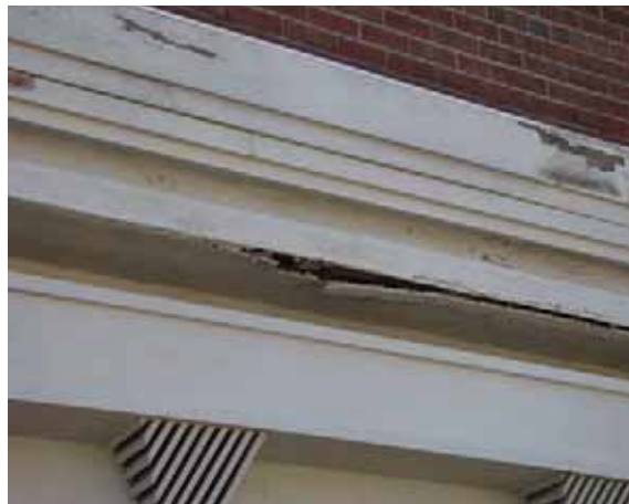
Left: Rotted soffit and fascia at 129 N Race.
