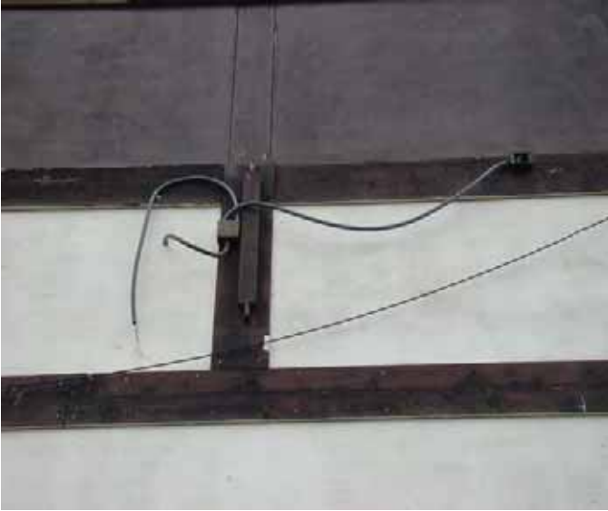
Above: Exposed and uncapped wiring at 201 S. Race.
