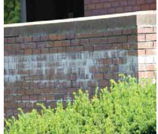
Above: The brick porch and stair section located at 202 S. Broadway is in need of tuck-pointing.
