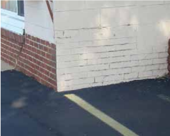
Left: A deteriorated brick wall at 403 N. Vine.
