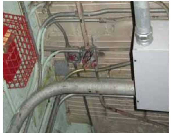
Right: Improperly terminated wires. (04/04/2016)
