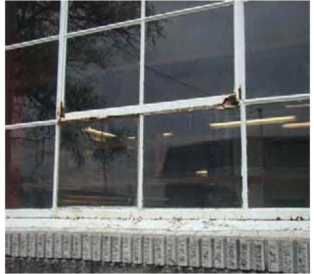
Right: The window muntins at 104 S. Vine are rusted.
