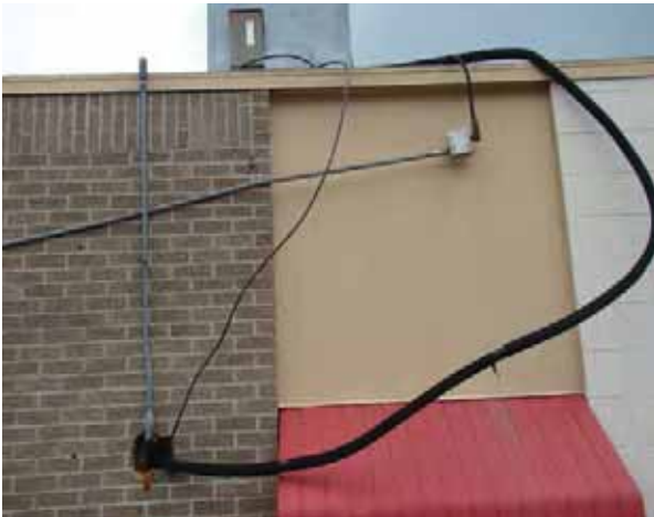
Left: Unsecured hoses and wiring conduit at 207 E. Illinois.
