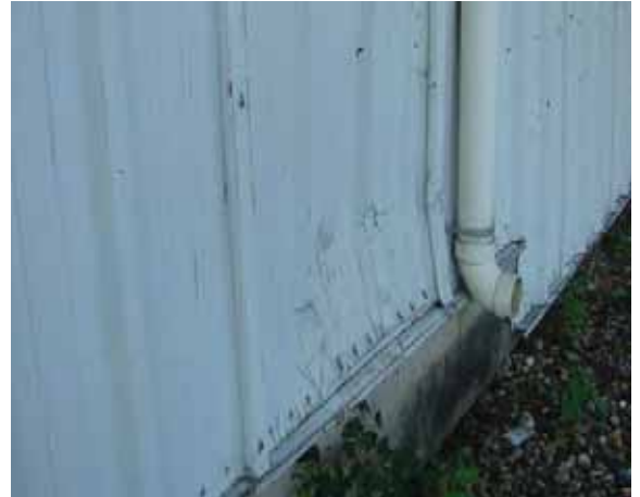
Right: The steel walls at 105 E. University are dented and deteriorated.
