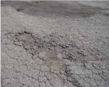
Left and Right: A deteriorated parking lot and curb stop located at 1501 N. 12th Street.
