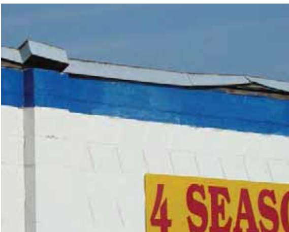
Left: Dislodged flashing at 401 N. Broadway.
