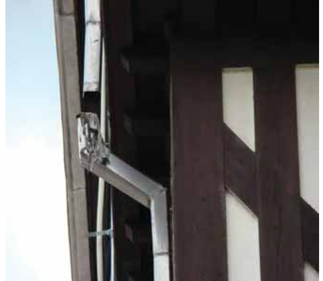
Above: A downspout at 201 S. Race has been dislodged.
