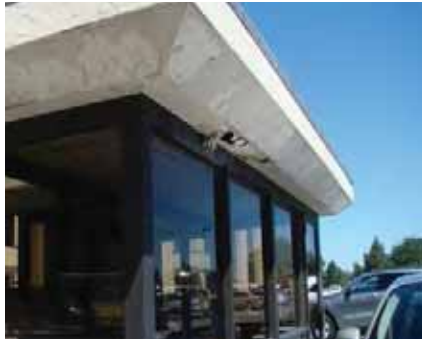
Right: The parking attendant building at 109 E. Walnut has a hole in the soffit.
