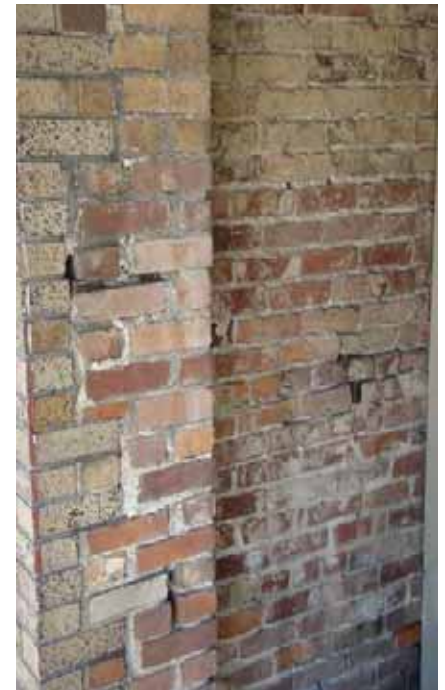
Below: Another example of the needed tuck-pointing at 110 W. Main.
