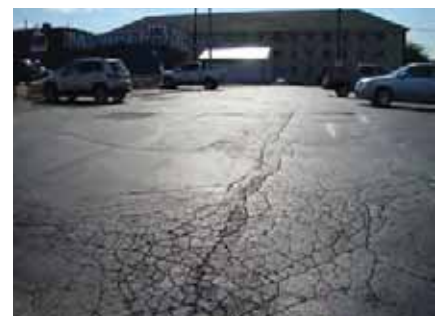
Above: The parking lot at 710 W. Florida Avenue has severe alligator cracking.
