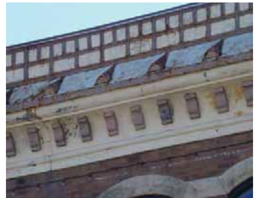
Above: The exterior tin cornice at 122 S. Race is rusted.
