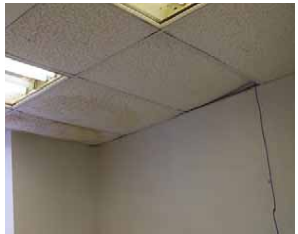
Right: Interior water damage at park building 901. (03/08/2016)
