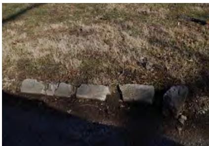
Left and Right: The curbs and gutters in Crystal Lake Park are deteriorated. (03/08/2016)
