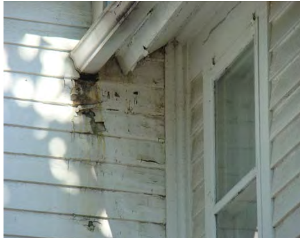
Right: The wood siding on 206 S. Cedar has rotted due to water leaking from the gutter.
