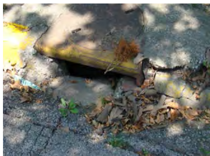
Above: A deteriorated storm drain along California Avenue.
