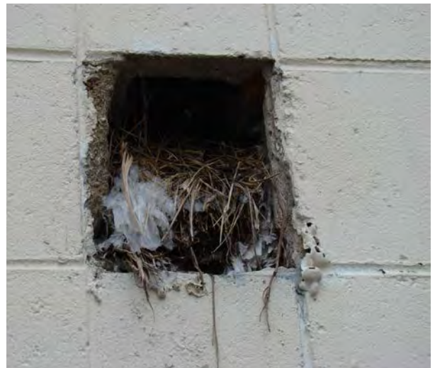
Right: A nest in an uncovered hole in the exterior wall at 207 E. Illinois.
