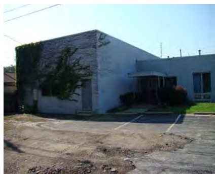
Left: The rear lot for the above property along Vine Street is also deteriorated.
