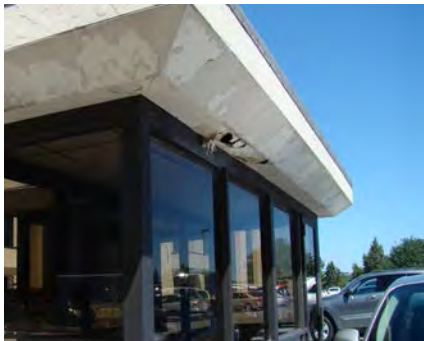
Right: The parking attendant building at 109 E. Walnut has a hole in the soffit.
