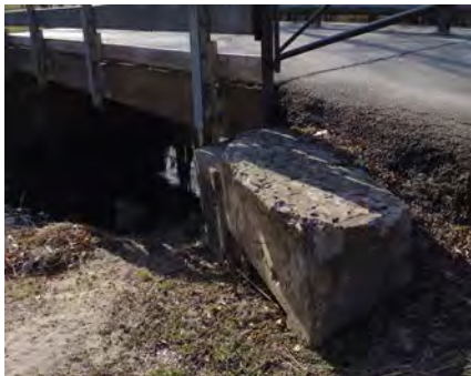
Left: The bridges in Crystal Lake Park are deteriorated. (03/08/2016)
