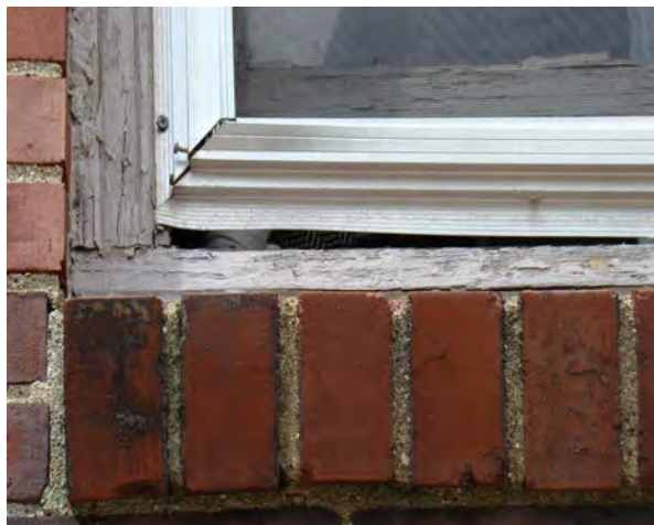
Right: The window frames at 402 S. Race are deteriorated.
