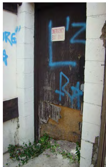
Below: Graffiti on a deteriorated door at 201 S. Race Street.
