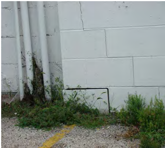
Left: Foundation settlement at 301 E. Main.
