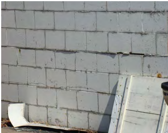
Left: Deteriorated mortar joints in the concrete block walls at 401 N. Broadway.
