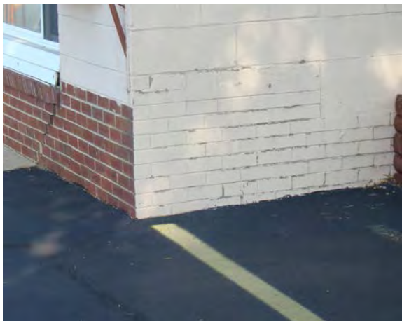
Left: A deteriorated brick wall at 403 N. Vine.
