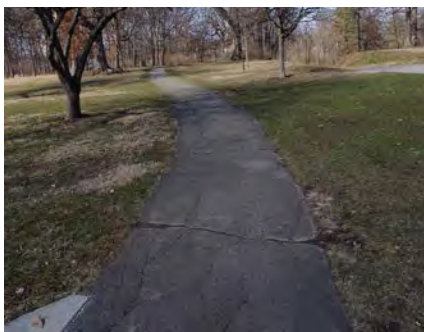
Left and Right: The pathway located in Crystal Lake Park is deteriorated. (03/08/2016)
