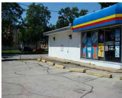
Above: A deteriorated parking lot located at 306 W. Water Main.
