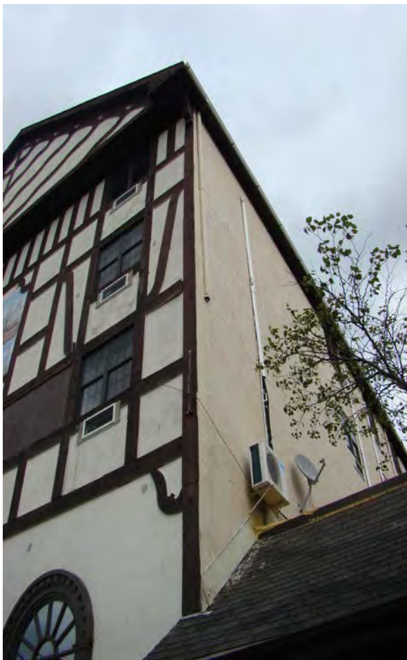
Left: A large portion of the downspout is missing at 201 S. Race.
