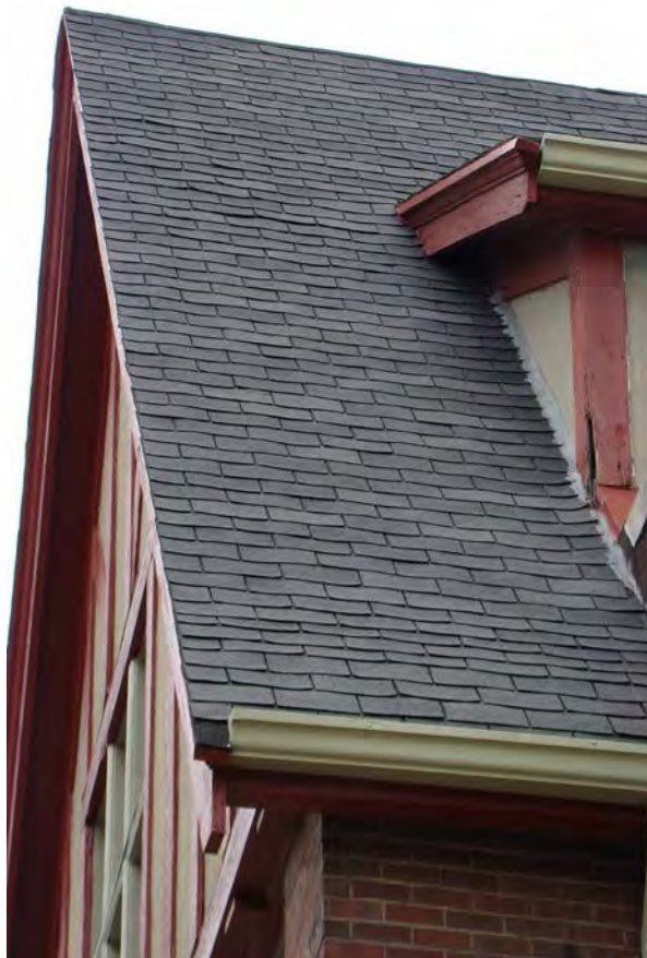
Right: The shingles on 402 S. Race are in need of replacement.
