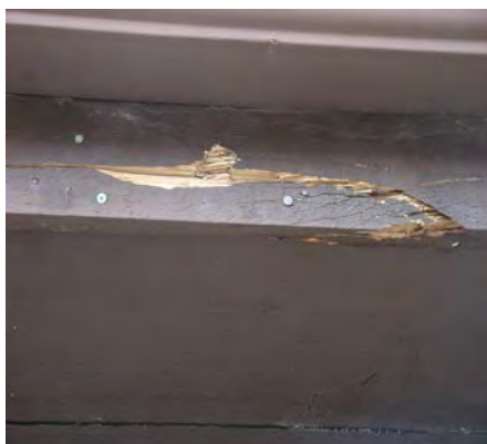
Below: The wood trim at 201 S. Race is deteriorated.
