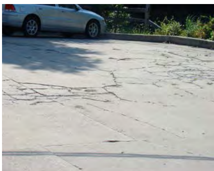
Left: The parking lot for 402 N. Broadway is deteriorated.
