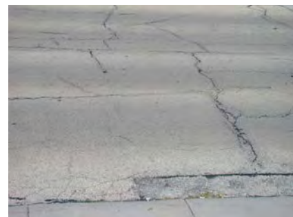
Above: Deteriorated pavement along Illinois Street.
