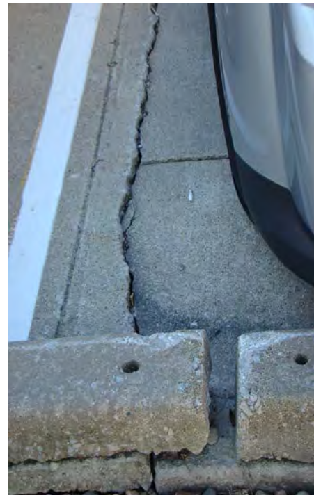
Above: A large shear crack, due to excess settling at 207 W Elm Street.
