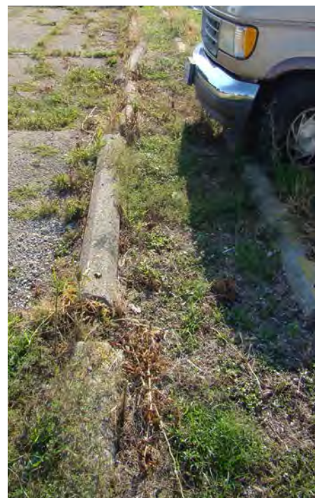
Right: 201 N. Broadway is a deteriorated public parking lot.
