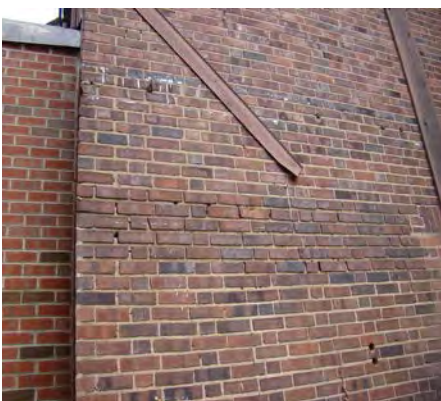
Below: The brick walls at 201 S. Race are in need of tuck-pointing.
