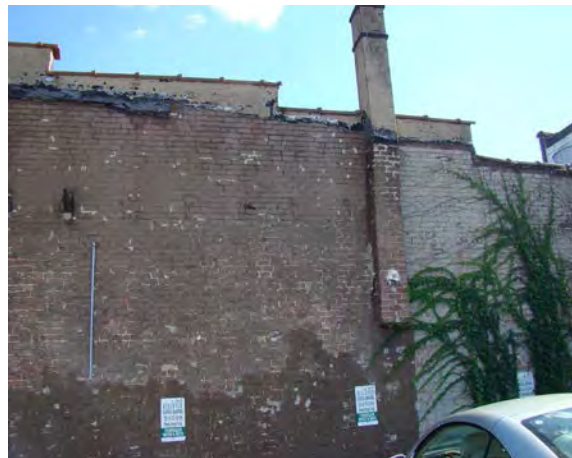
Right: The chimney and exterior brick wall at 201 N. Broadway are deteriorated.
