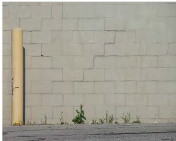
Right: Step cracking in the concrete block wall at 220 N. Broadway.
