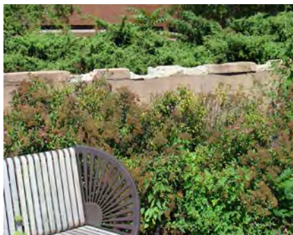
Above: This retaining wall located at 1776 E. Washington is cracked and crumbling.
