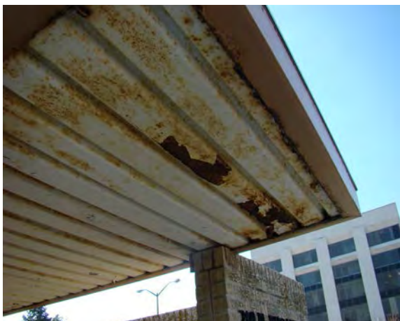
Left: The metal roof on 210 N. Broadway has rusted.
