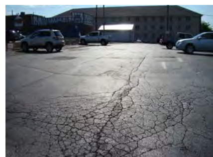
Above: The parking lot at 710 W. Florida Avenue has severe alligator cracking.
