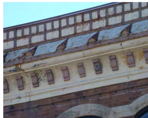
Above: The exterior tin cornice at 122 S. Race is rusted.
