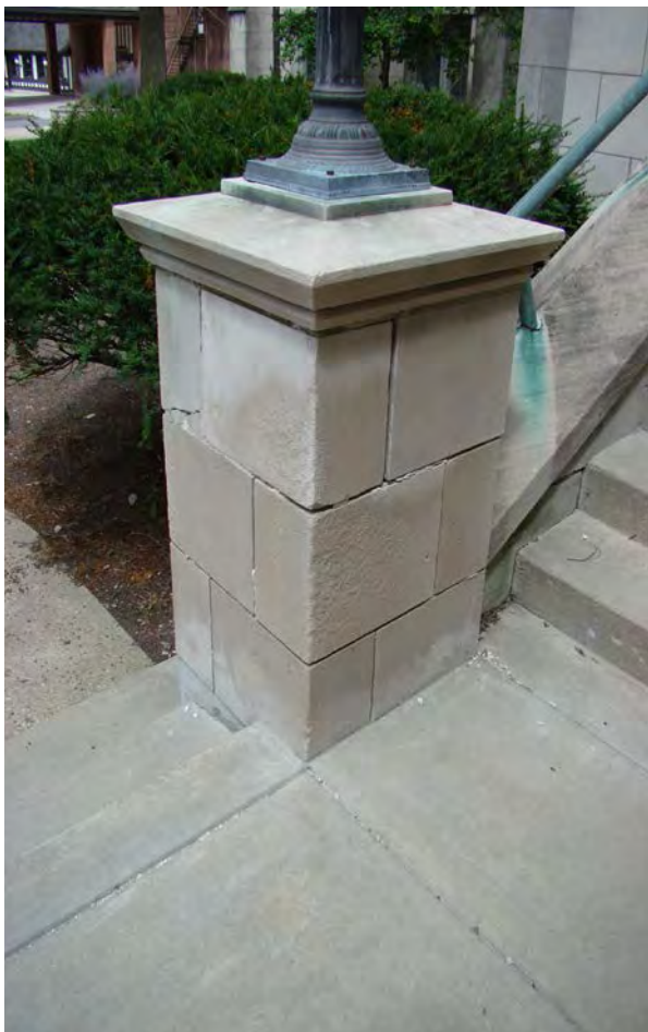
Left: The porch columns at 304 S. Race. are in need of tuck-pointing.
