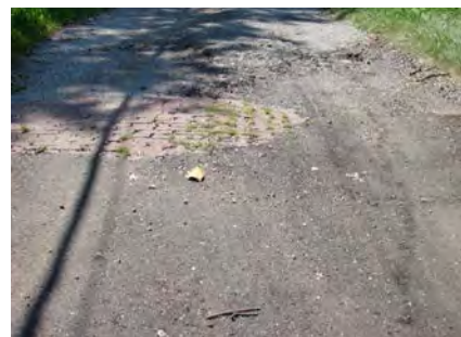
Below: This alley between Vine Street and Urbana Avenue is severely deteriorated.
