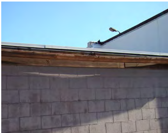
Left: A rusted and sagging gutter located at 201 W. Green.
