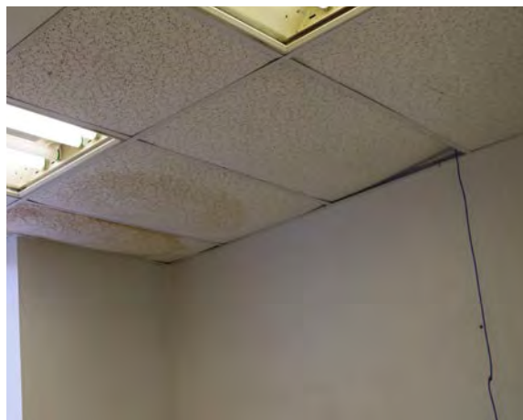
Right: Interior water damage at park building 901. (03/08/2016)
